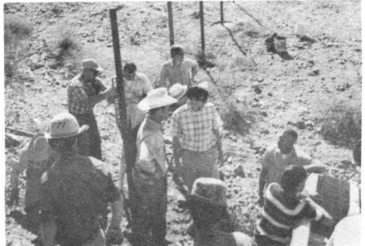
As is typical with any large project, problems are encountered along the way. Here John Houzenga (center, with white hat) and Harry Hazlett (leaning on the back of the truck) are consulting how to solve a construction problem. All problems were solved and the project was finished in record time. Both photos on this page by Cecil La Vance.
