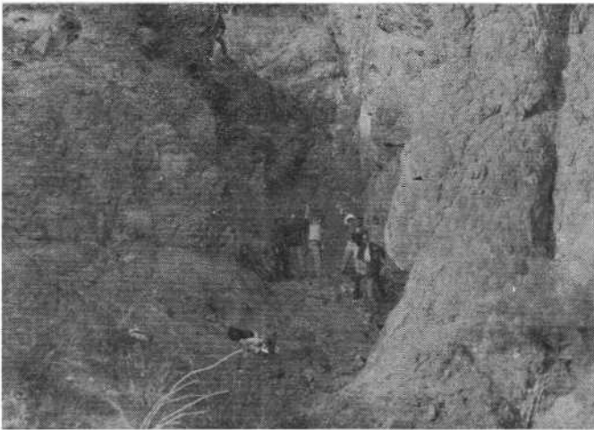
Members of the Society start work to prepare the site where the dam will stand. Left to right: Carl Scrivens, Frank Murphy, Terry Evens, Jerry Petkovsek, Joe Kane and John Houzenga.
