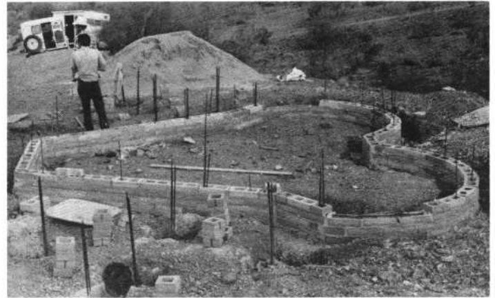
This remarkable photograph shows the foundation of our exhibit building and its resemblance to a ram's head. The two gents in upper left are Ed Shannahan and John Houzenga. All photographs by Doug Reynolds.
