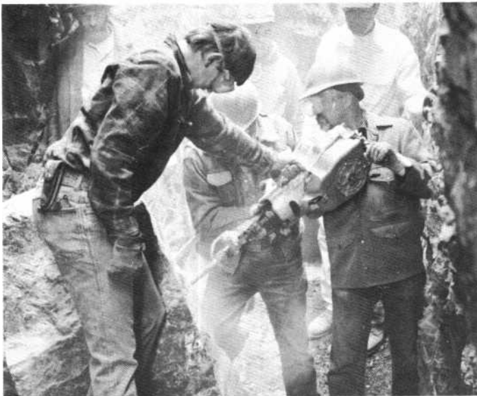
The portable jack hammer was invaluable in busting up these large boulders. Bill Snider, Yuma is the operator with Dave Mitchell helping to steady the hammer. In background from left to right Keith Gundry, Joe Gundry and Bob Gray.
