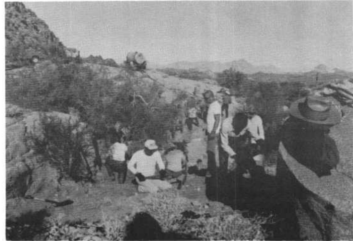
Construction of a small diversion dam on the west side of the tank.
