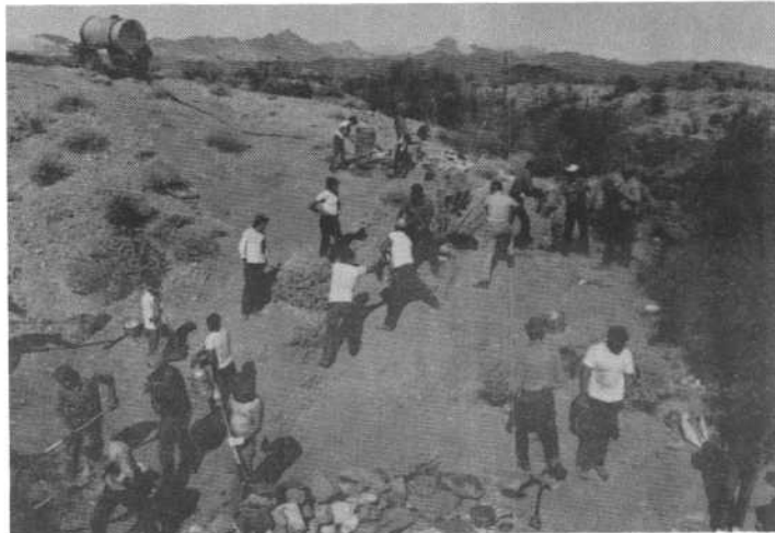
Our clean-up crew excavating silt and debris between the two rip-rap dams. Note the bucket-brigade operation.
