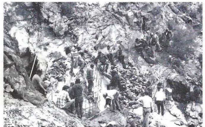
Masonry dam begins to take shape. Note rebar core. Anvil Tank, February, 1980.
